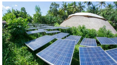
Şekil 13. Green School, güneş panelleri ( https://inhabitat.com/green-school-in-bali-shows-students-how-to-live-sustainably/ )
