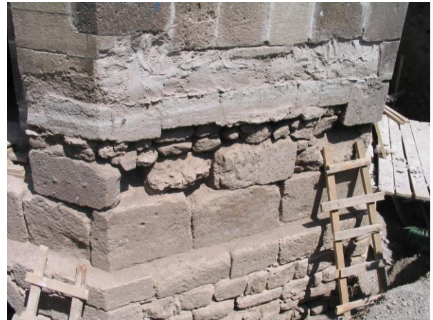
Figure 5. The historic building damaged wall surface made by bricks belonging to Seljuk Empire.
