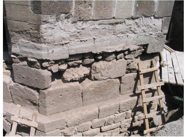
Figure 5. The historic building damaged wall surface made by bricks belonging to Seljuk Empire.
